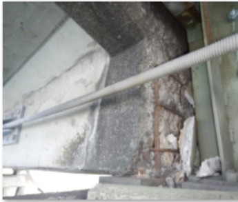
26211-A Girder 17A end spalling with exp rebar (4).JPG
