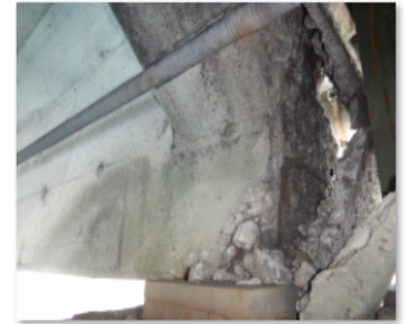
26211-A Girder 17C end spalling with exp rebar (2).JPG
