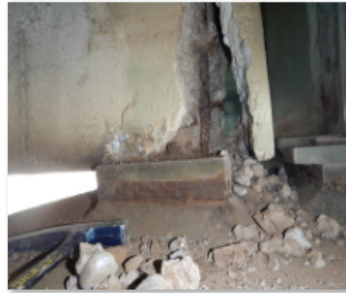
26211-A Girder 17B end spalling with exp rebar (3).JPG
