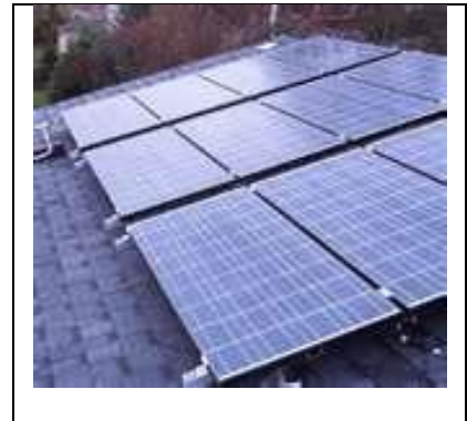
Figure EE-2 Solar Panels, the New Face of Power Generation
