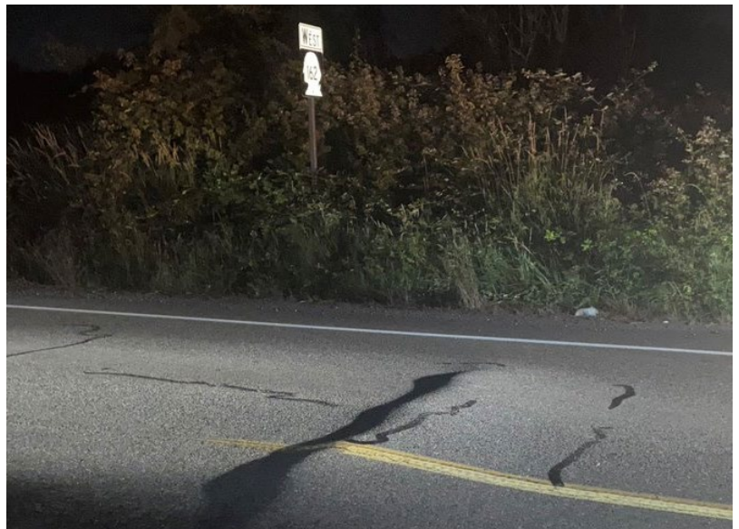
Between June 26-28, 2021, temperatures reached 107°F in South Prairie causing the pavement along SR 162 to warp and elevate nearly four inches. Source: WSDOT
